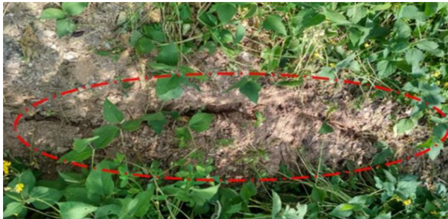
Figure 5: Ground distress due to tunneling.
